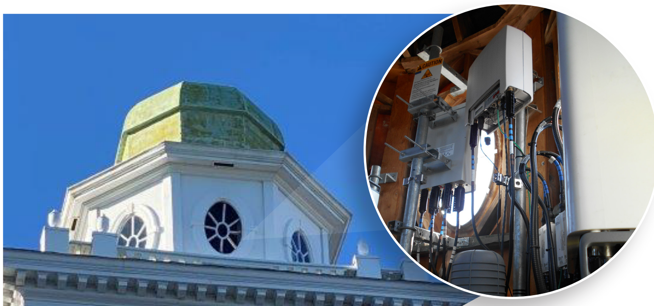
Figure 2: Massachusetts Cupola concealing 5G equipment.
