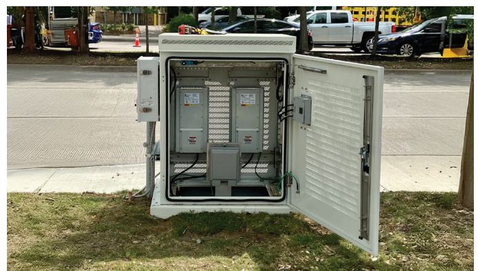
Figure 2: Ground Cabinet Enclosure
