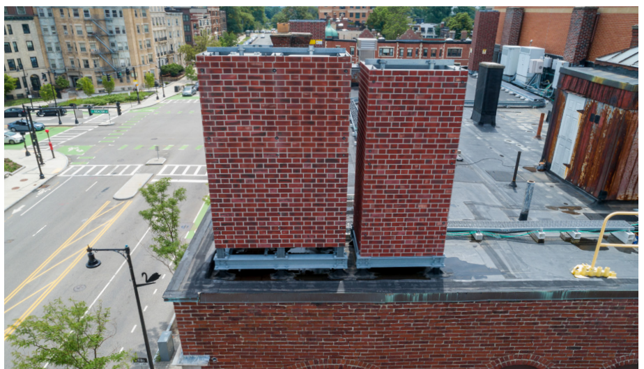
These rooftop macro cell sites use Raycap's SSV/ESSV panels and SSV/ESSV with InvisiWave apertures to conceal the wireless radio equipment inside.
