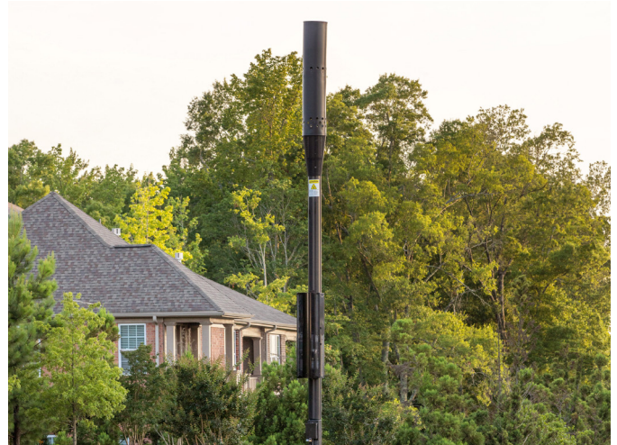
Figure 1: Streetlight poles are an obvious option for urban small cells, and the top of the pole provides the best line of sight for 5G coverage.
