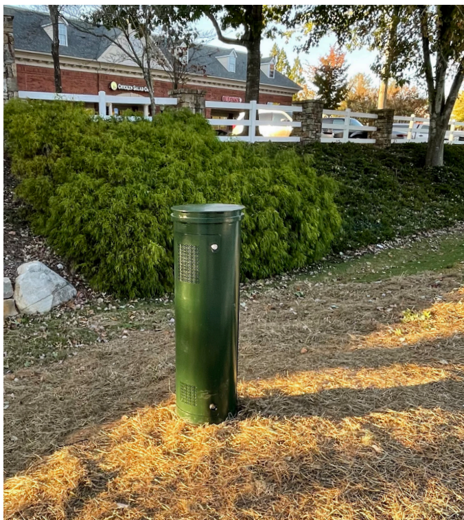
Figure 4: Cylindrical ground furniture can place support electronics up to 20 feet away from a pole with mounted 4G/5G radios.
