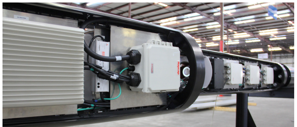
Figure 1: AC power and equipment compartments in an integrated 5G small cell pole assembly.
