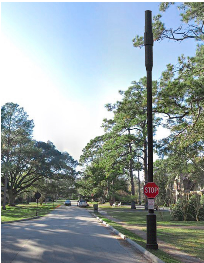
We designed this integrated small cell pole to provide 5G mmWave service around the Houston, Texas area.
