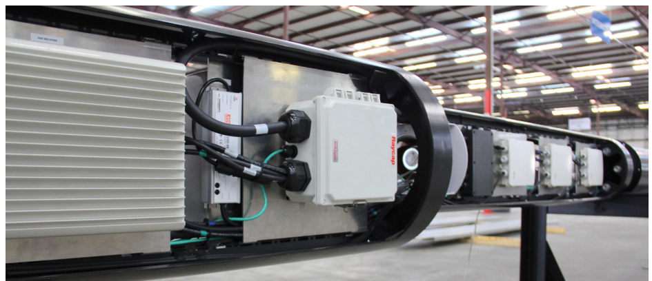
Figure 1: AC power and equipment compartments in an integrated 5G small cell pole assembly.
